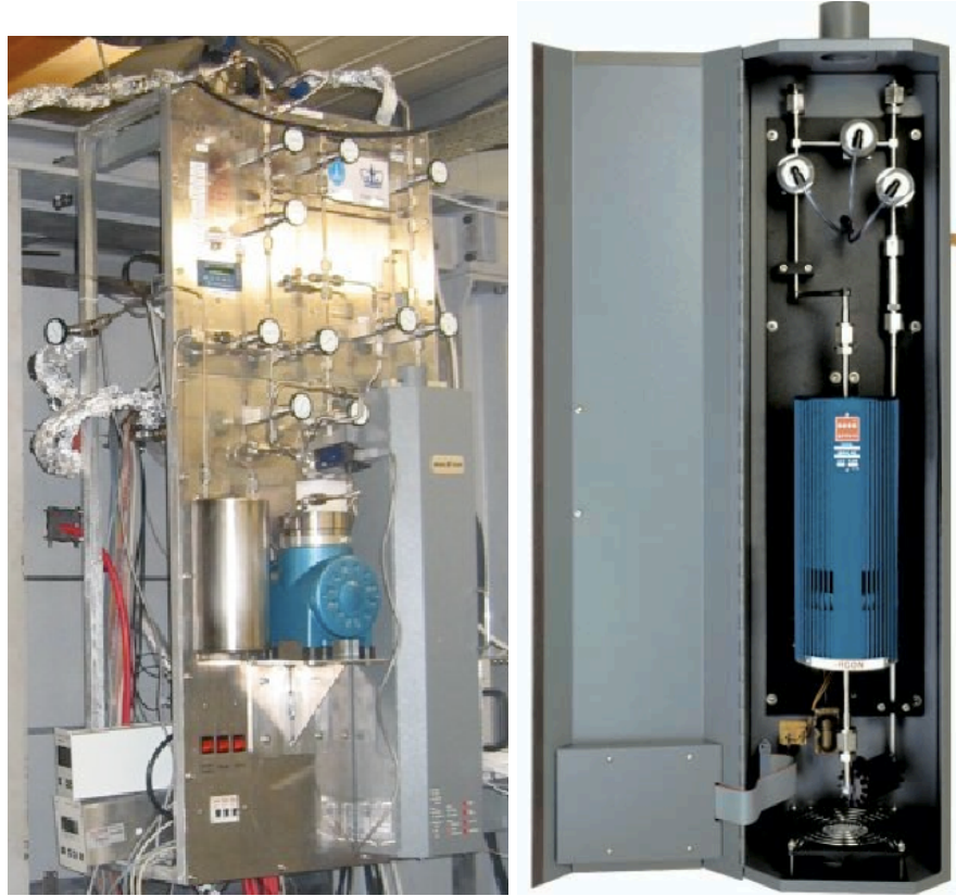
Figure 3.25: (left) The Xe gas handling & purification panel, mounted on the XENON10 shield door. (right) Close-up of the SAES PS4 high-temperature getter.
