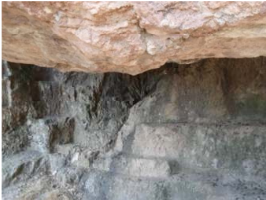
Fig. 5.30 Interior of Grotto with water channel along the west wall (right) with water stains on the stairs (left) (author photo)
