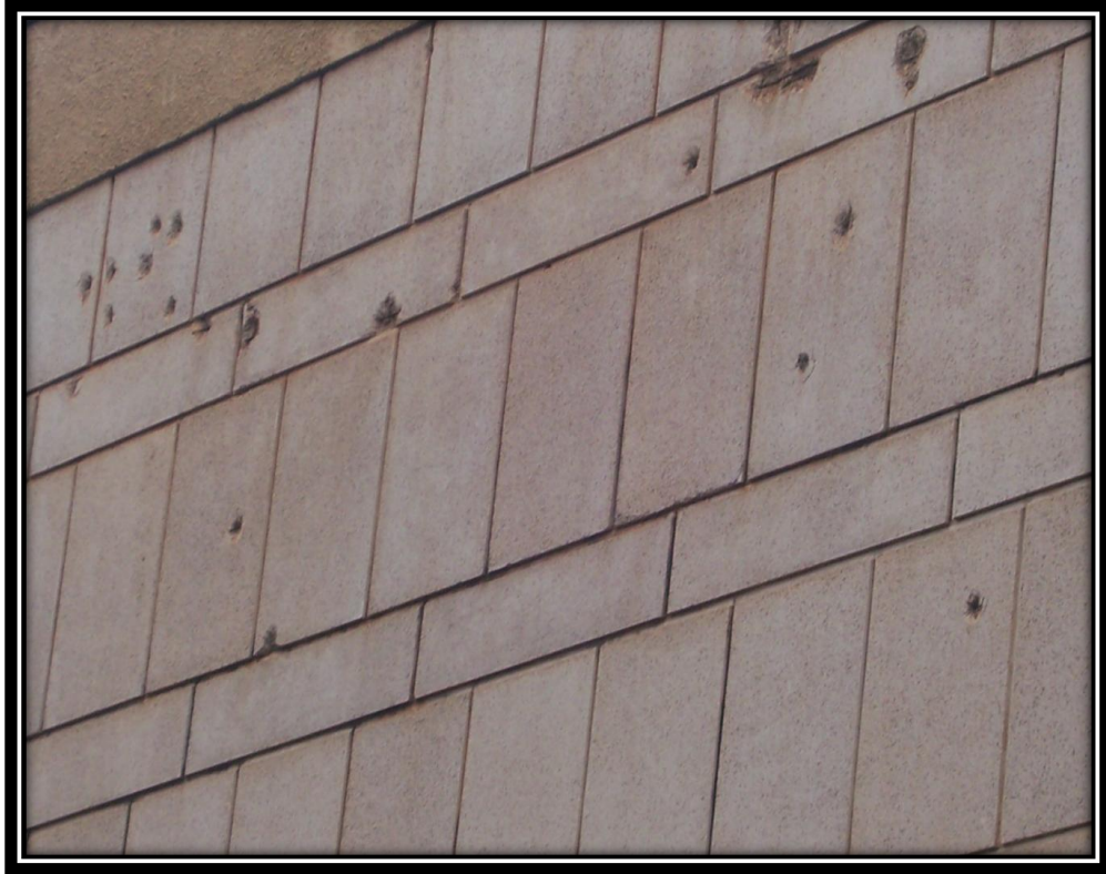
8. National Theatre, Uganda: Bullet Holes on the Walls, 2007. The bullet holes on the walls, however, were recently erased during renovations appended to the Commonwealth Head of Government Meeting (CHOGM) event (November 2007) and, by extension, the Queen of England, Elizabeth II's, visit.
