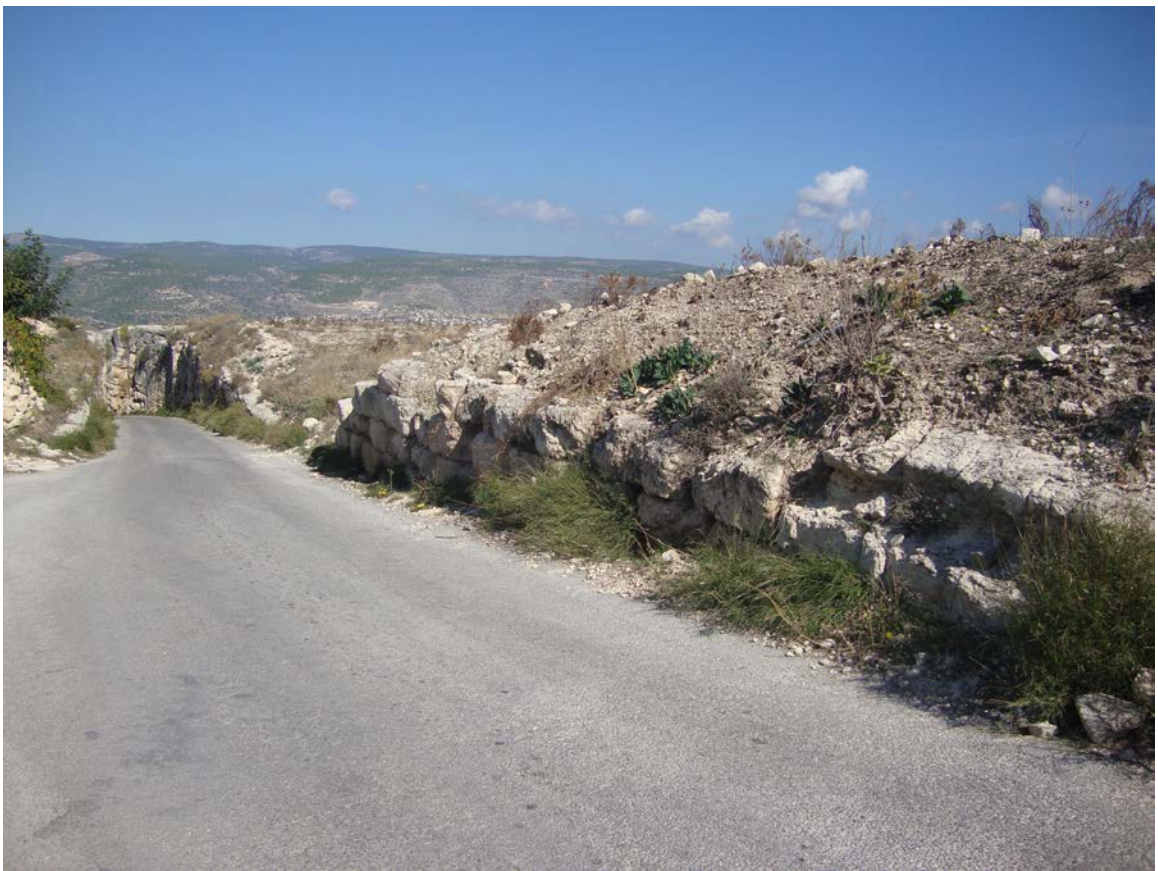
Fig. 5.28. Hagia Thekla. Additional blocks used to shore up the continuing walls of the rock-cut road north of the complex towards Seleukeia.
