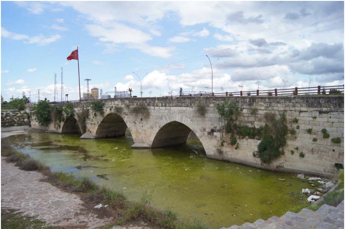
Fig. 5.11. The bridge at Tarsos (cf. Hild and Hellenkemper 1990: Abb. 378, which shows the visible part of the bridge before the alluvium was cleared).
