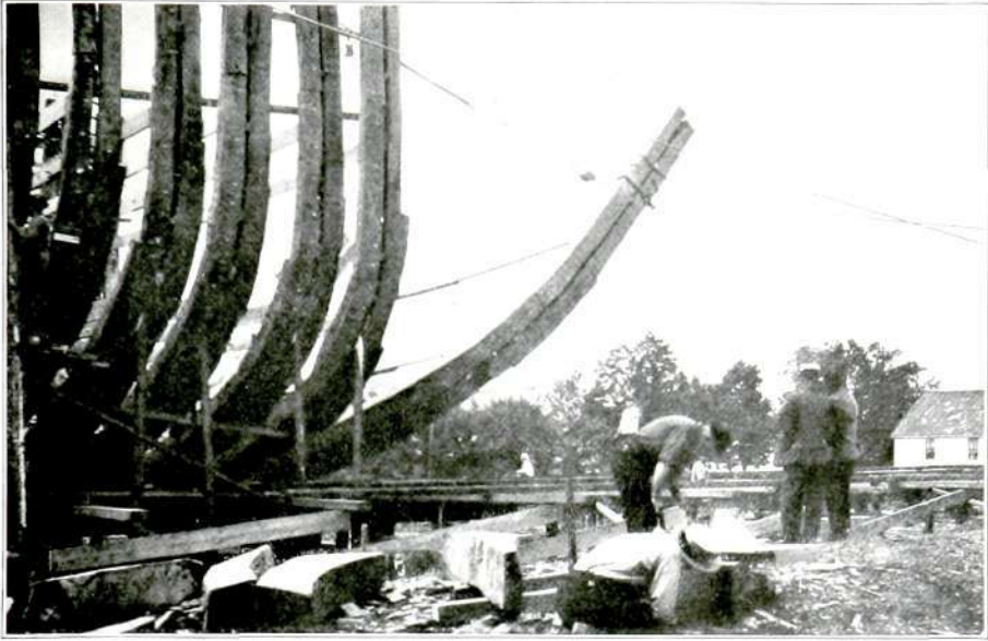
Hoisting the frame into place with block and tackle, Bean's yard, Camden, Maine. They work in wood for the love of it, hand and eye wonderfully trained.—Page 564.
