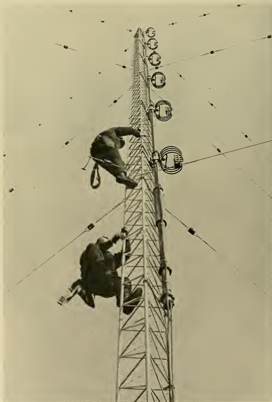
A TOWER FOR WBRU-FM: The signal from the Campus has a 40-mile radius.
